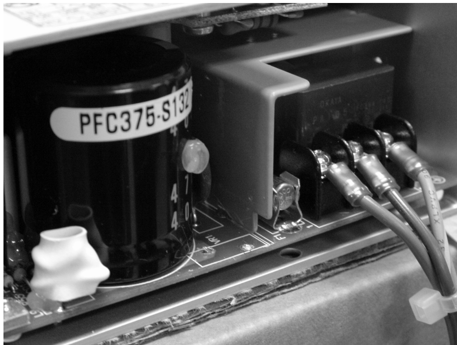
Figure 2: rear view of the power supply, MOV (VR1) has been removed
