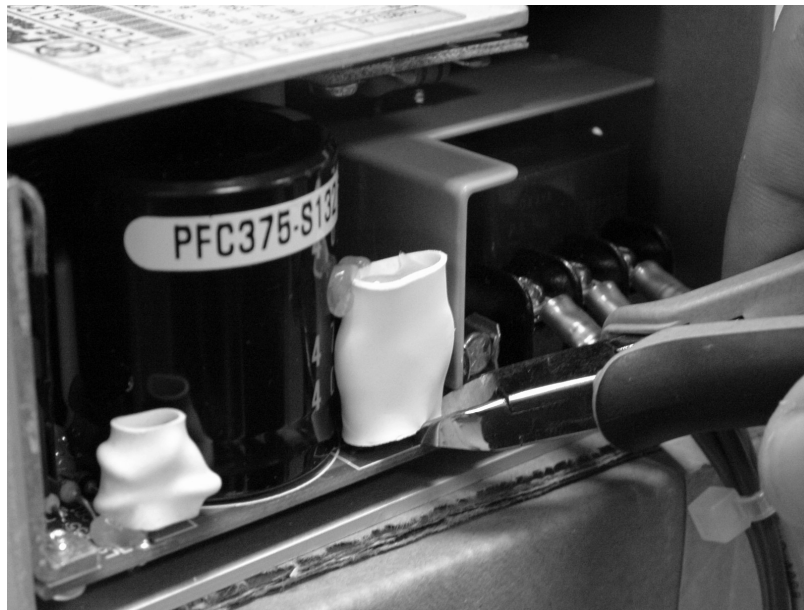
Figure 1: MOV shown while being removed by use of wire cutting pliers
