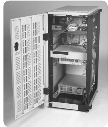
Figure 5.4. Rear-mounting the switching subsystem reduces rack space and minimizes cable lengths
